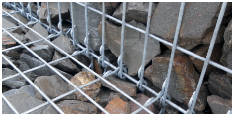
No protruding wire ends
